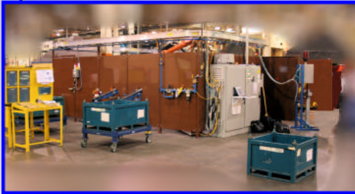
Robotic mig-weld system Installed at the customer
